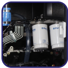
Fuel particle separator filter
