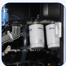
Fuel particle separator filter
